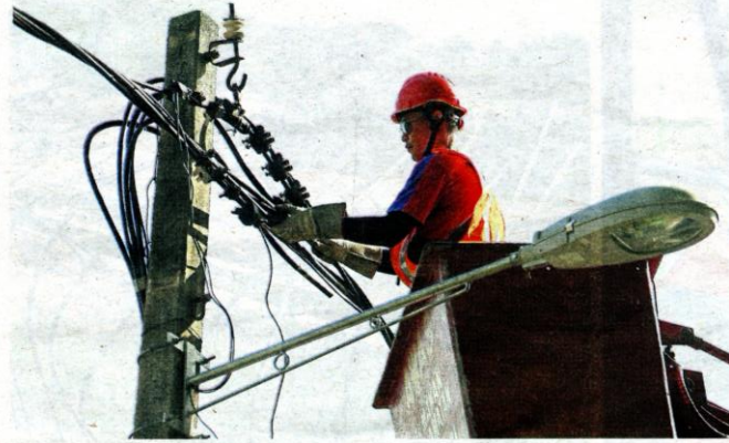
A TNB technician replacing the electric cables and joints in Jalan 17/46, Petaling Jaya.
